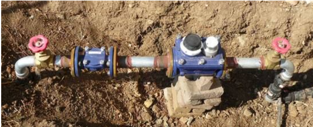
A connection to the municipal water supply with meter and stop cocks
